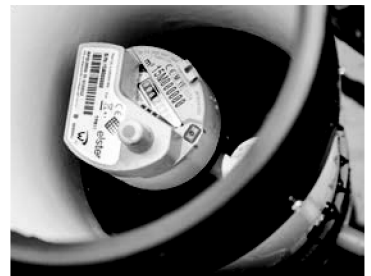
Meter in position
