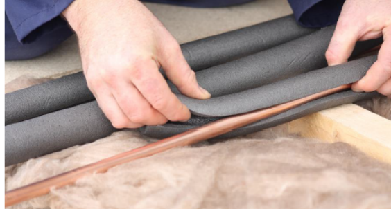
Insulate your pipes in cold places
