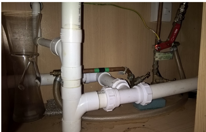
Figure 1 – Cross connection between rainwater and wholesome supply
