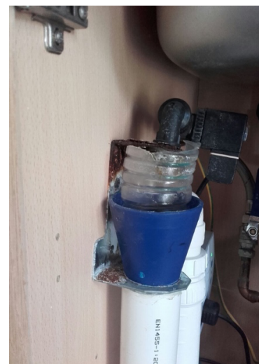
Figure 2 - Tundish with air gap obstructed
