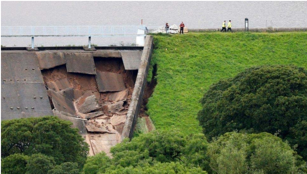
Figure 13 - Toddbrook Reservoir - spillway failure - 2019
